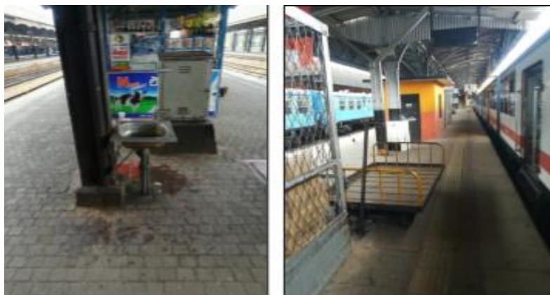
Figure 2: Improperly Built Drinking Water Fountain and Platform Deck Colombo Fort and Maradana Stations
